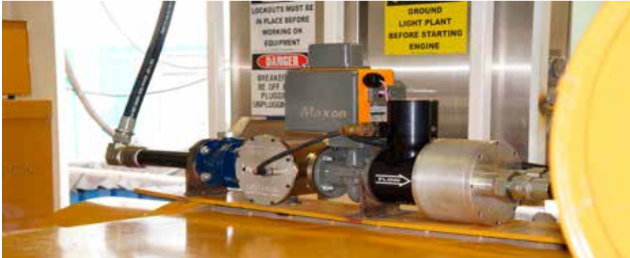
Typical Flanged Gas Train Assembly
